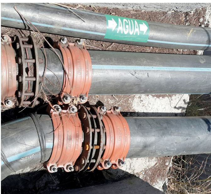
Thermo-fusion HDPE joint with a stub-end, plus counter flange and reinforced Victaulic 995 couplers
